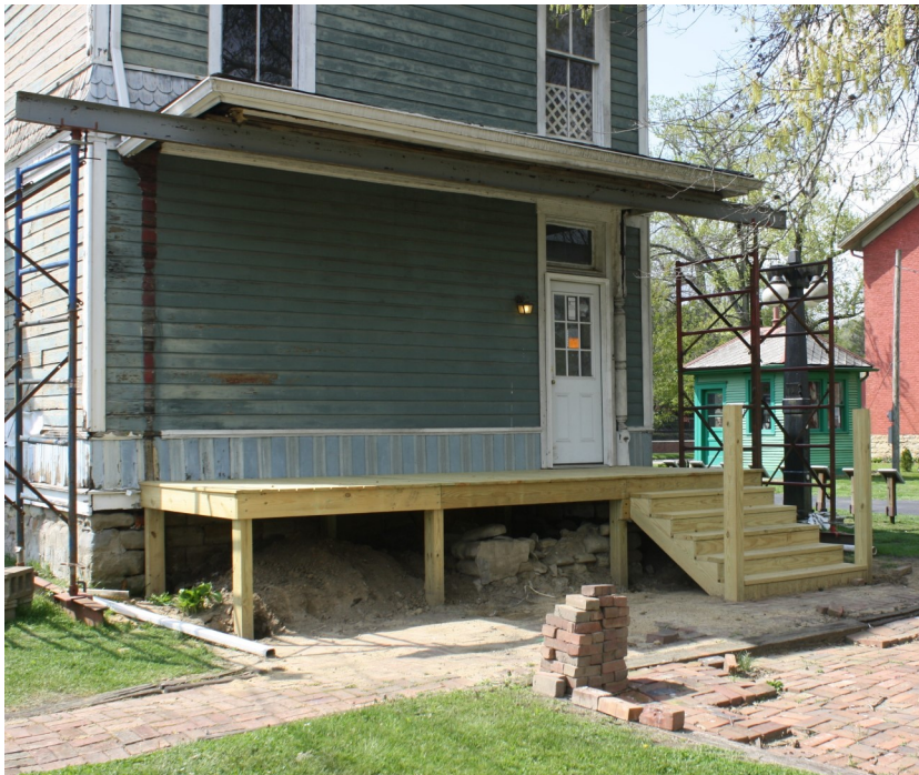
New back porch, sturdy enough to serve as a stage. New columns are being hand-turned from full dimension stock. The old entrance to the basement may be seen under the porch.
